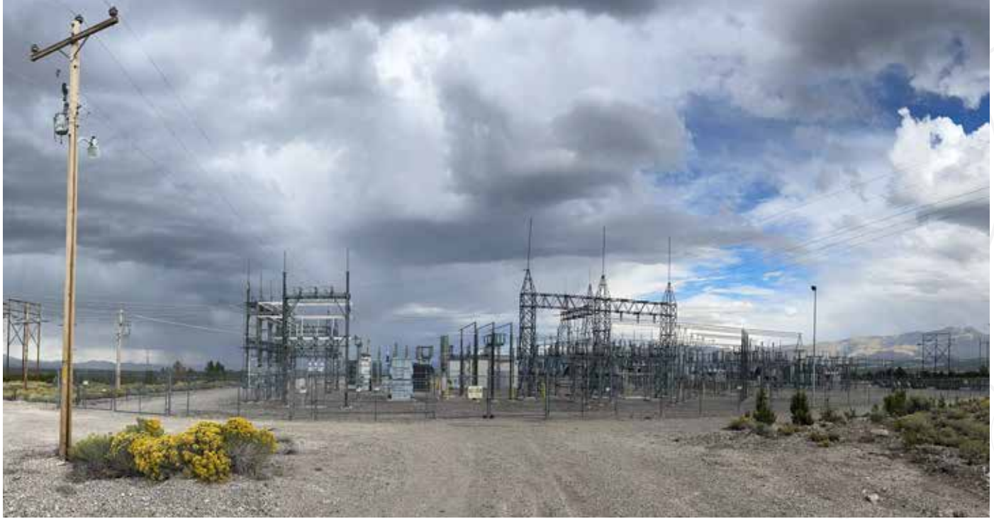
Figure 4. Machacek Substation. Source: Peter Gower/TNC.
